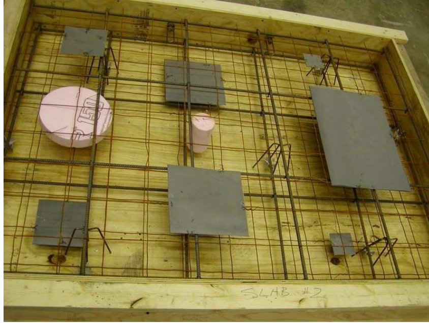
Figure 7.7: Photo of the form for slab No.2 containing artificial delaminations and voids.
